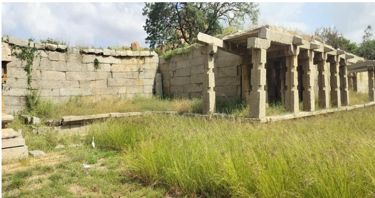
Before cleaning the vegetation at Achutadevaraya Temple at Venkatapura
