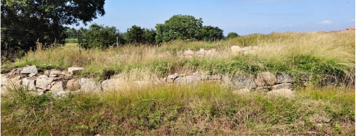
Before cleaning the vegetation at the Sasivekalu Ganesha Temple at Krishnapura
