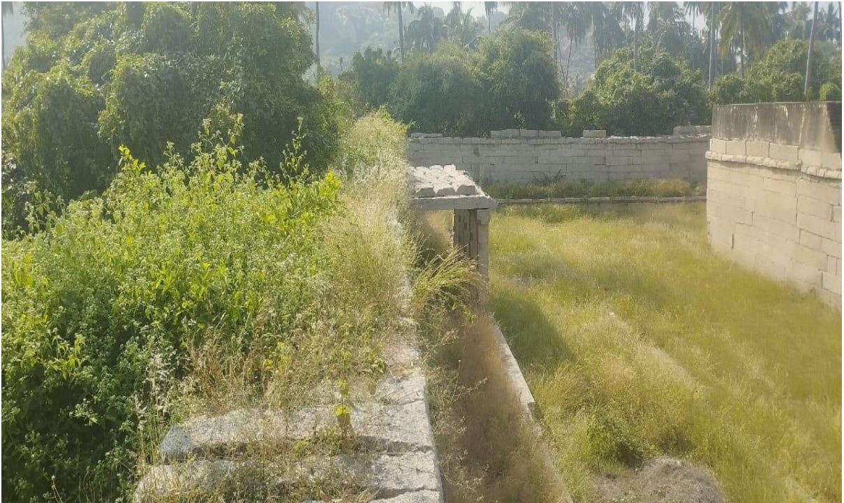
Before cleaning the vegetation at Achutadevaraya Temple at Venkatapura
